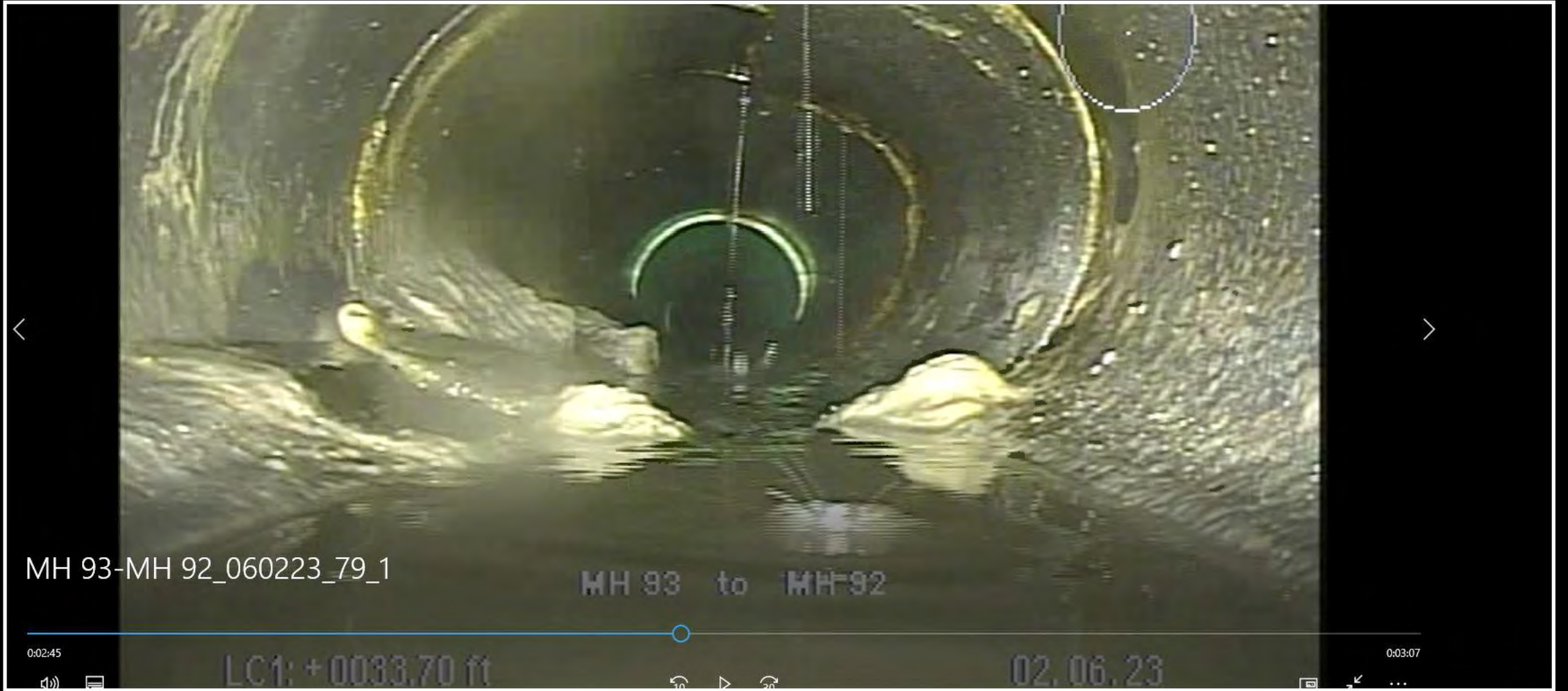
Lateral Crack, Leak, Crushed
