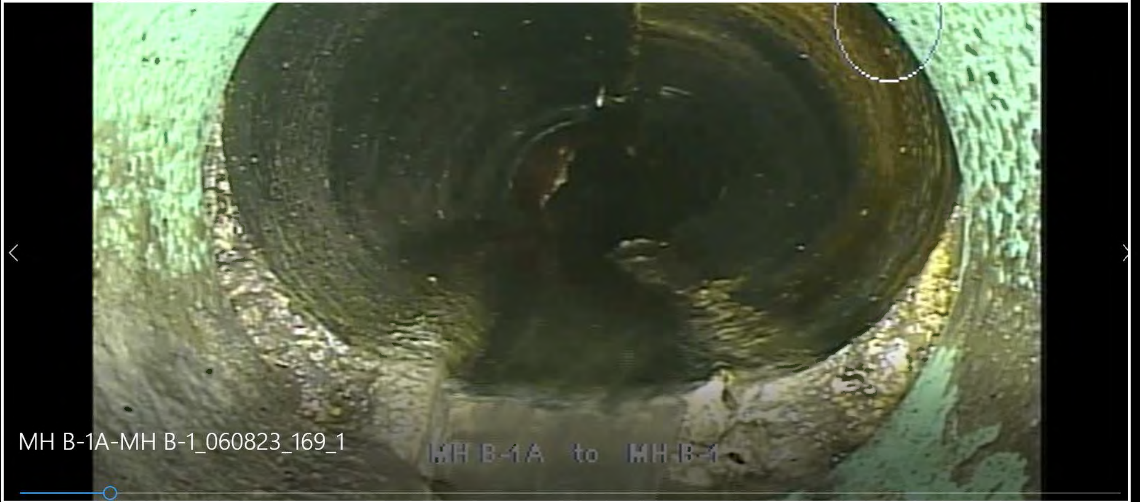
Crushed Pipe, Lateral crack leading to 5
