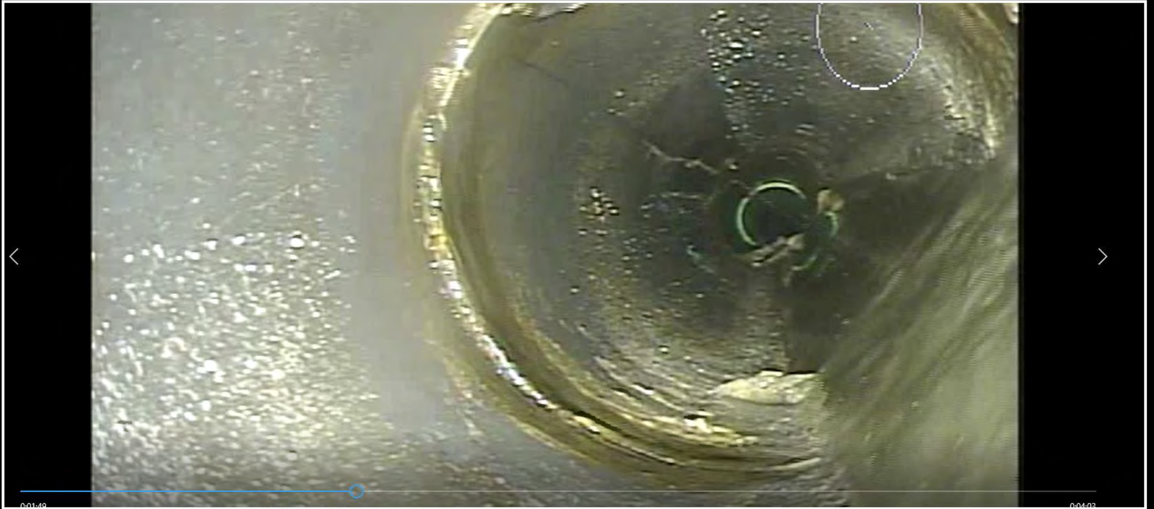
Lateral Crack Leaking Leading to 3
