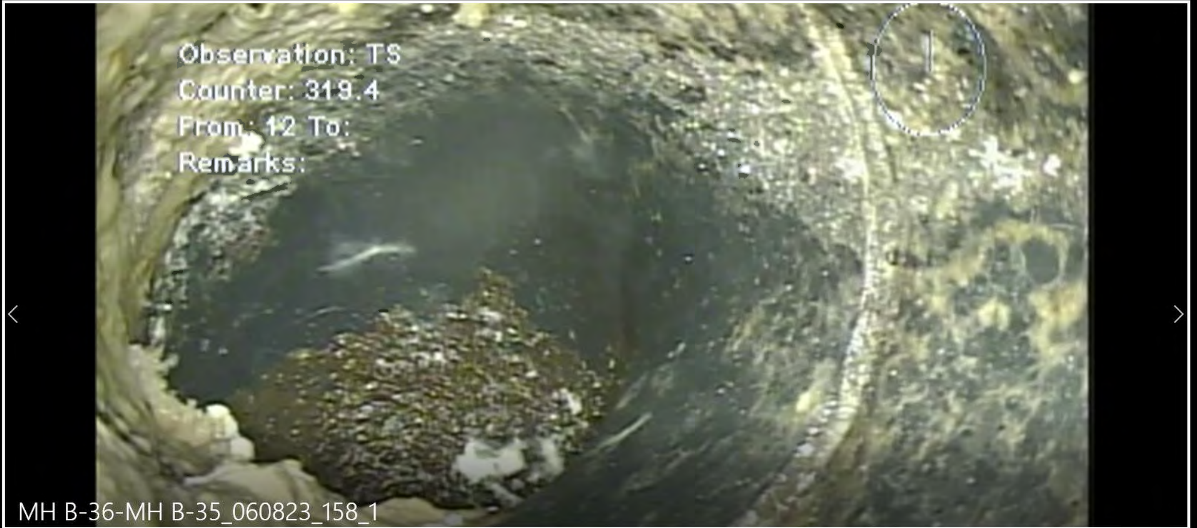
Grease In Lateral
