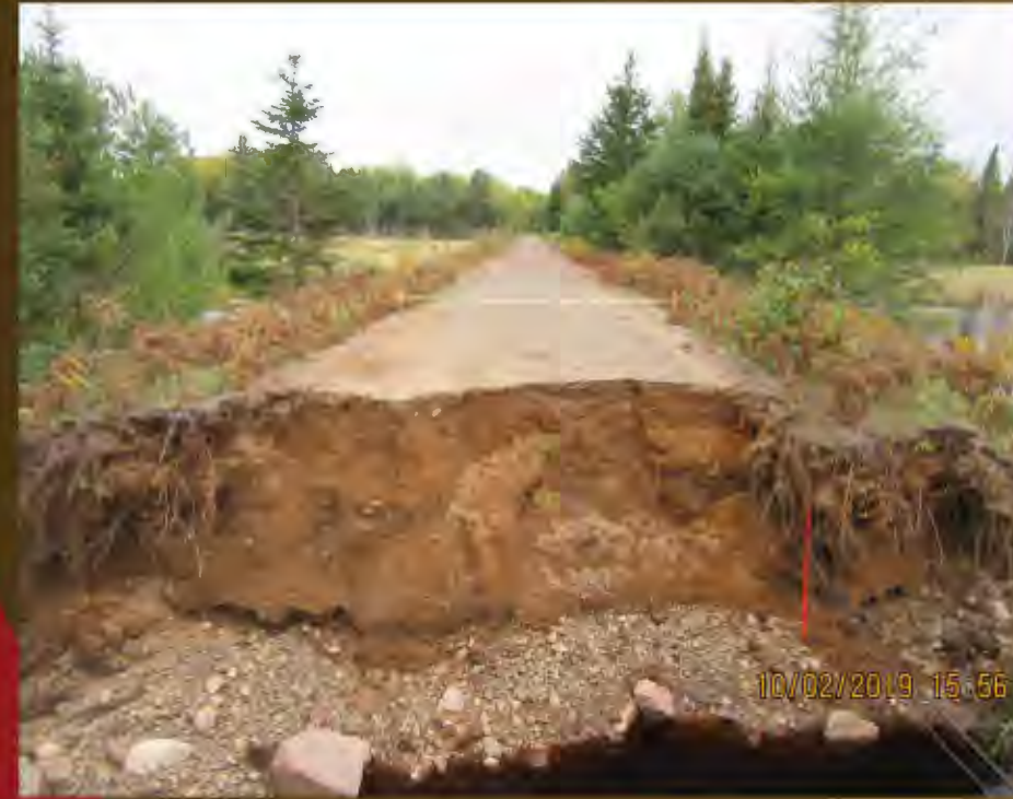
Fixed major culvert washout along with bridge replacement in Humboldt Township repaired with ORV funding
