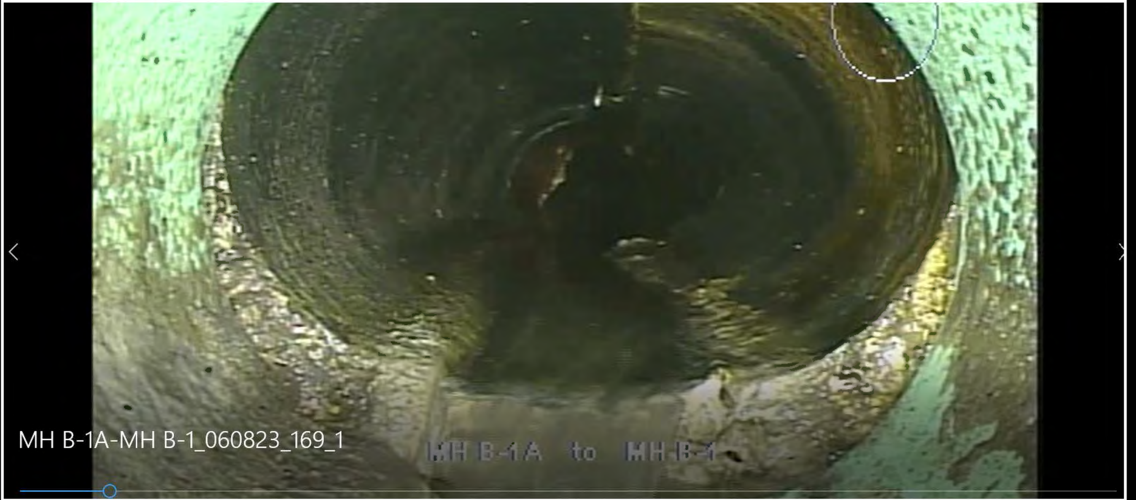
Crushed Pipe, Lateral crack leading to 5
