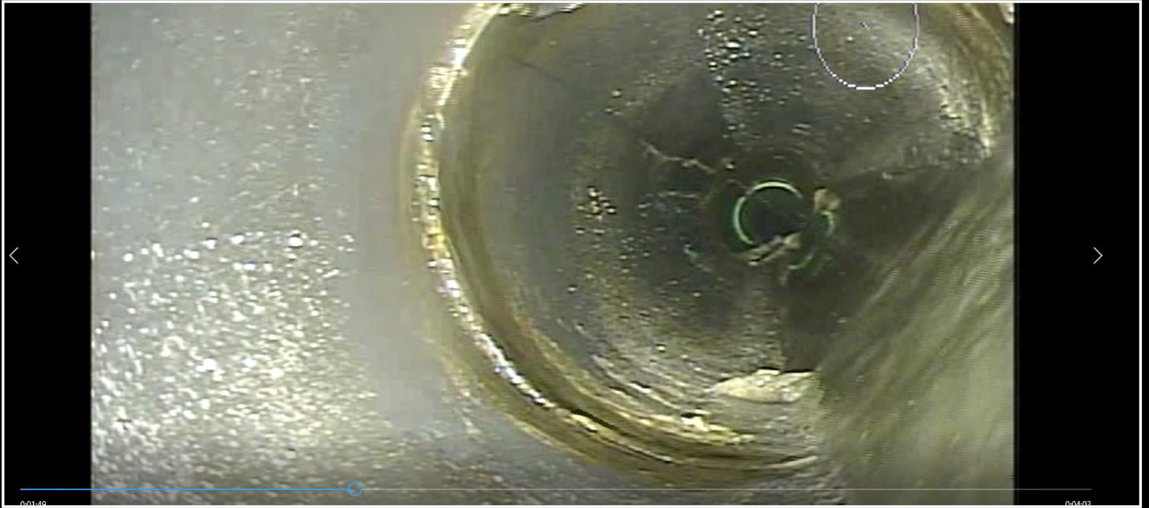
Lateral Crack Leaking Leading to 3
