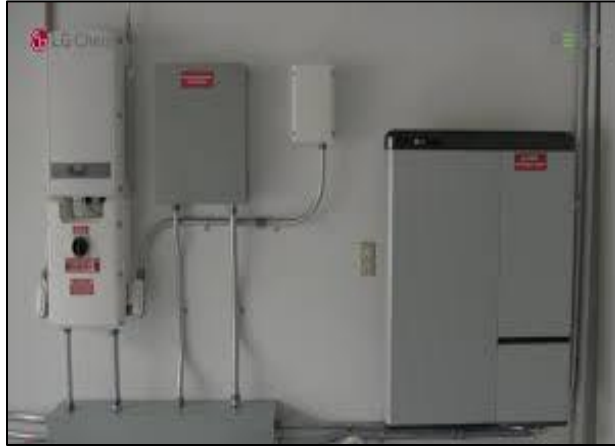
Example power storage system
