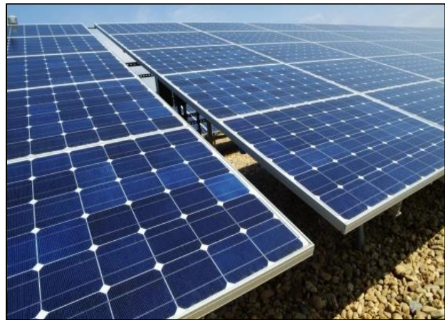
Marquette Board of Power and Light solar array
