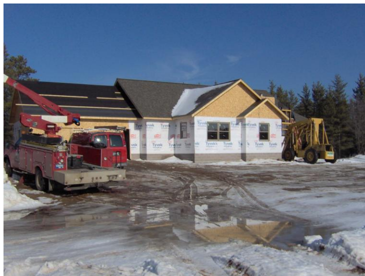
Photo 1-1 Chocolay Township is Likely to Experience a Significant Portion of Marquette County Growth
